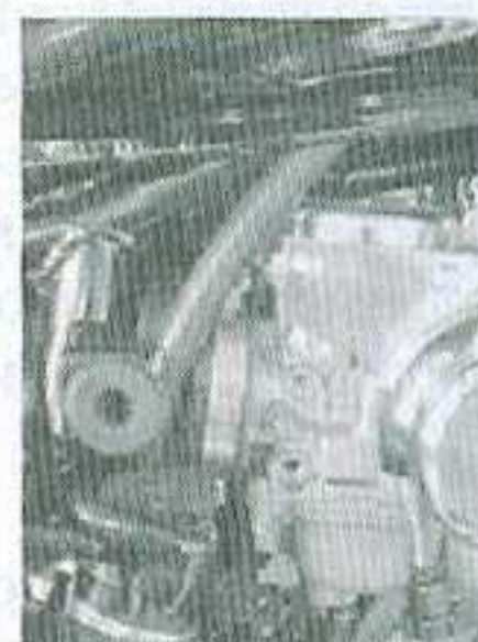
③ water pipe
