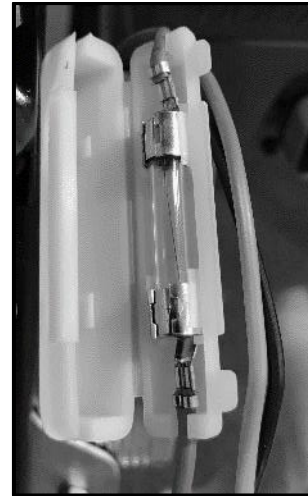
Converter fuse and its holder opened
